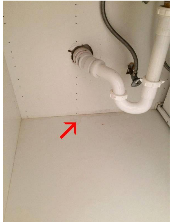
Staining-Dry at time of Inspection
