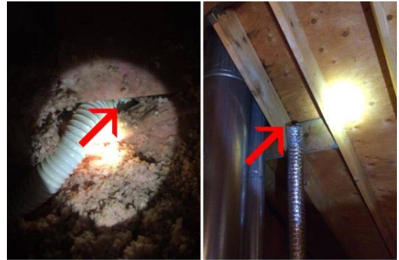
Exhaust Fans Discharge in Attic
