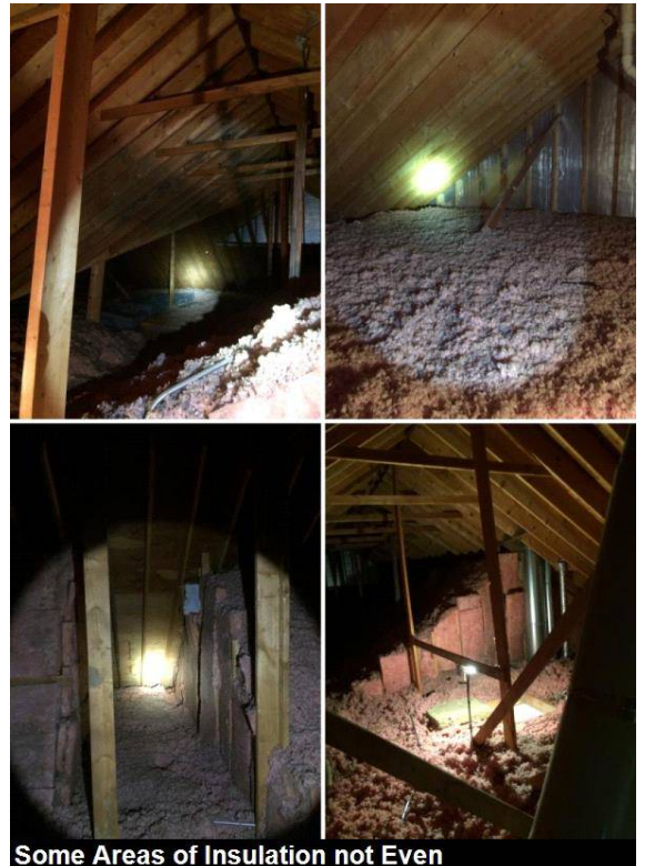
Some Areas of Insulation not Even
