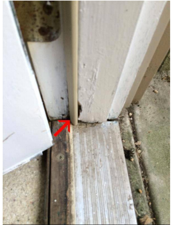
Rotted Side Jam, Basement Exterior Door
