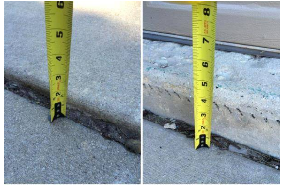
Trip Hazard at Garage Lip
