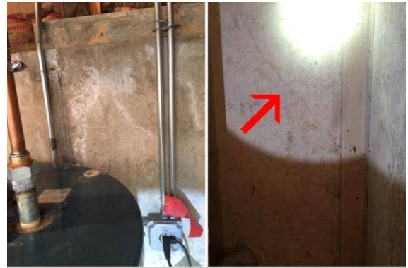
Common Cracks / Efflorescence
